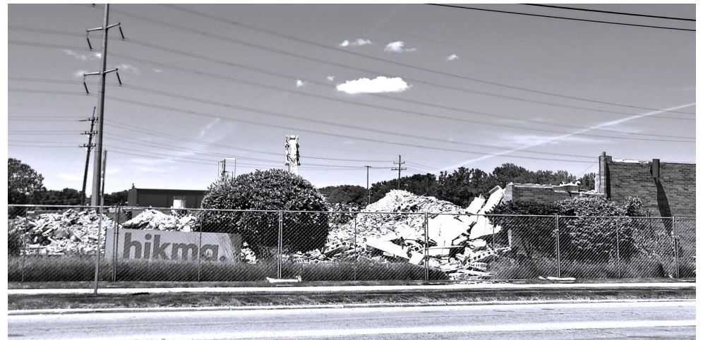
Construction continues at the Hikma plant on Northfield Rd., on a new warehouse for the company, as part of an expansion project at its Bedford facility. Photo by Elena Psenicka
