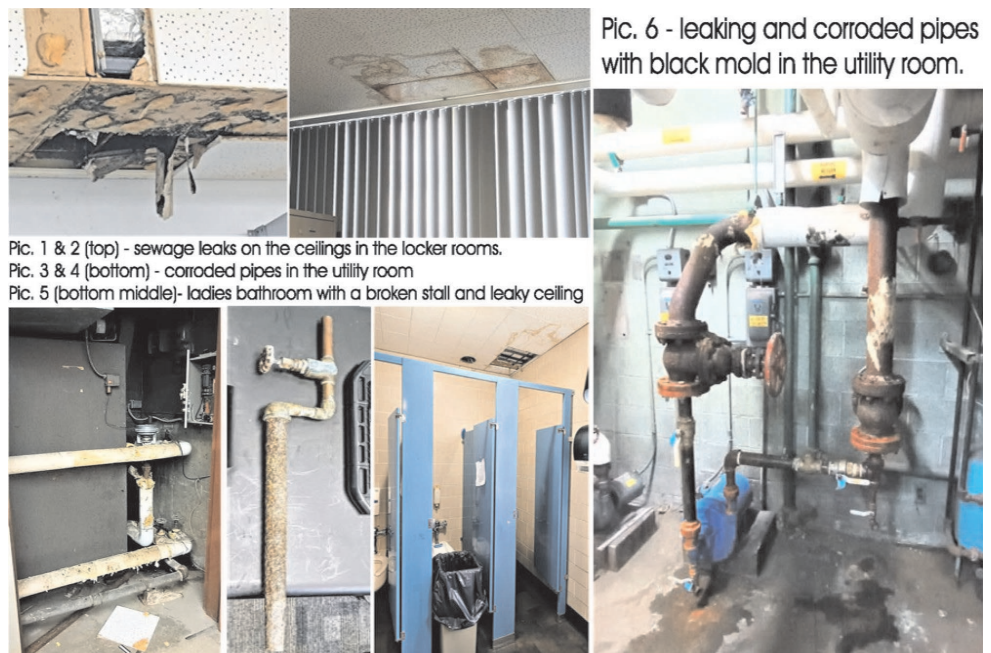
The Neighborhood News reported the deplorable conditions in the Justice Center building that houses the Garfield Heights Municipal Court, police station and jail in a 2022 news story that featured these photos taken above by Elena Psenicka.
