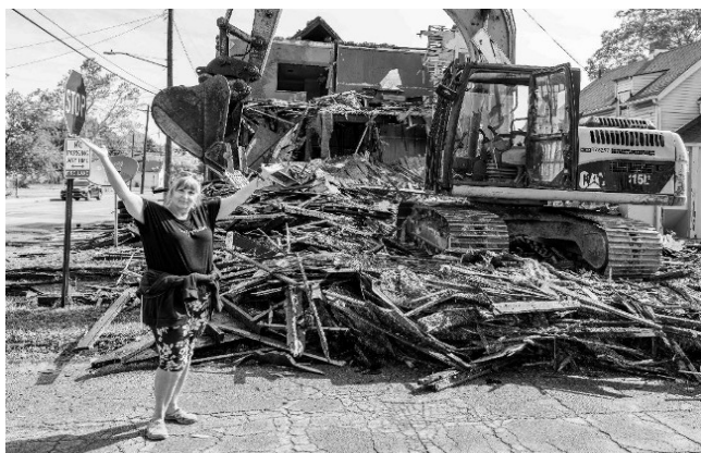
A member of Forest City Block Club celebrates the demolition. Photo by Mark Silverberg
