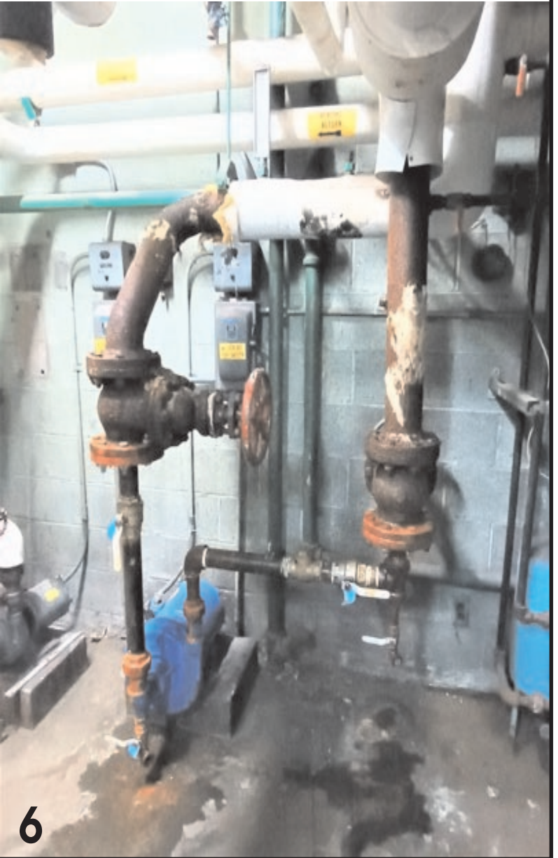
Pic. 6 - leaking and corroded pipes with black mold in the utility room.
