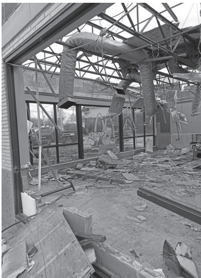
The McDonald's restaurant on Turney Rd. in Garfield Heights was demolished last week to make way for a new McDonald's on the site. Both McDonald's restaurants in Garfield Heights have the same owners.
