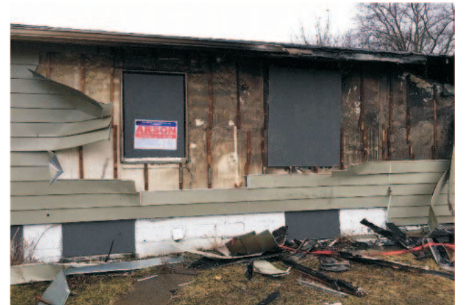
Above is the aftermath of an intentionally set fire at 719 Northfield Rd., Bedford.
